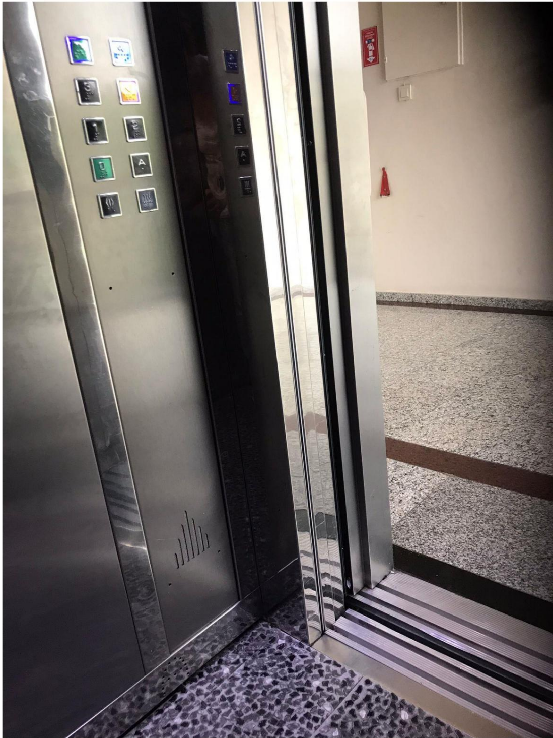
Disabled-friendly elevator in Vocational School Building
