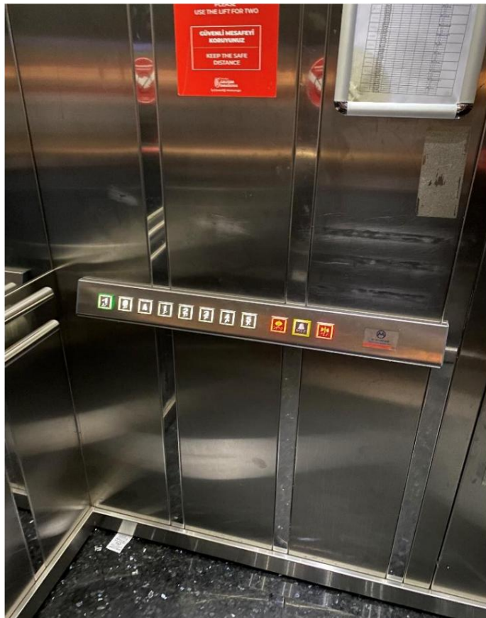
Images from our disabled-friendly elevators in Block A
