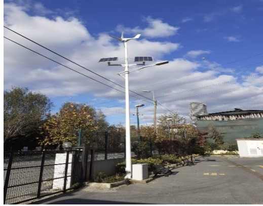
Figure 5. Block D environmental lighting pole powered by solar and wind energy
