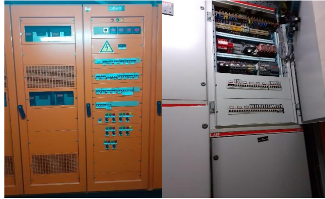
Figure 4. The MCC and DDC panels of Tower Campus
